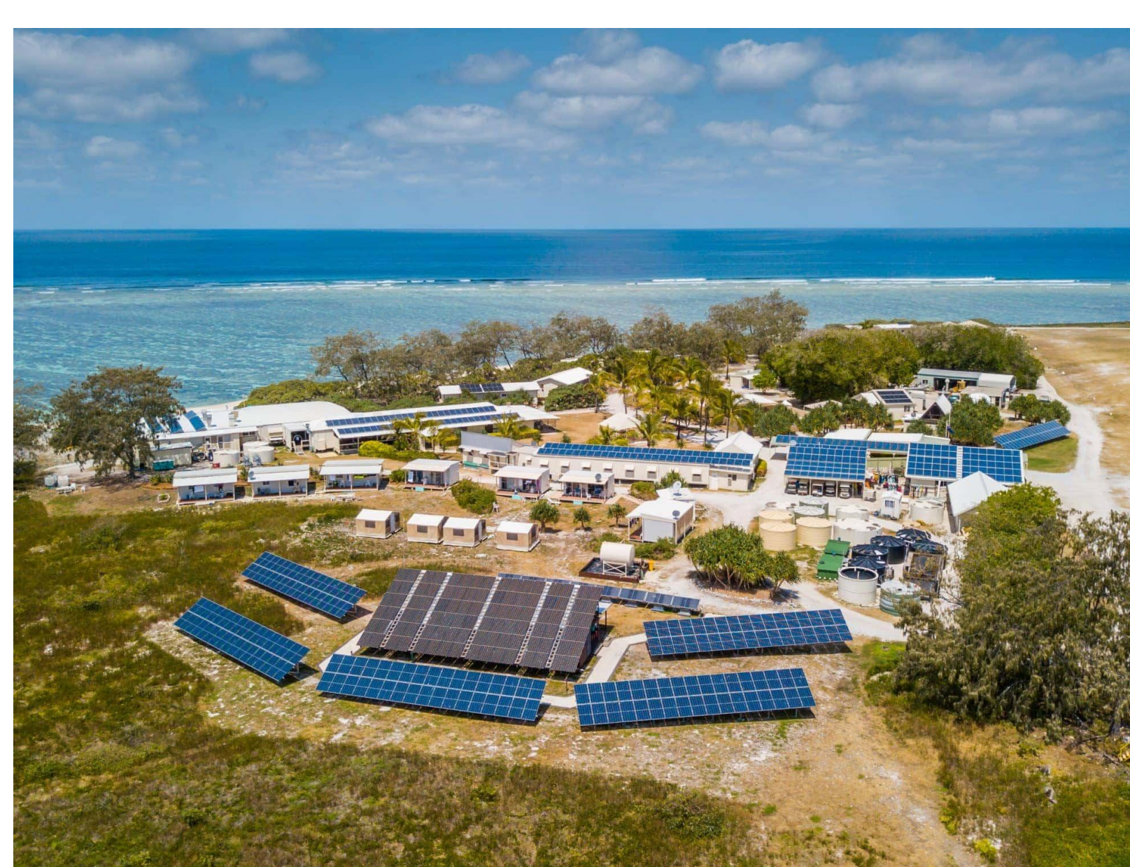
Lady Elliot island moving towards full sustainability (Qld, Aust.) – solar and battery
