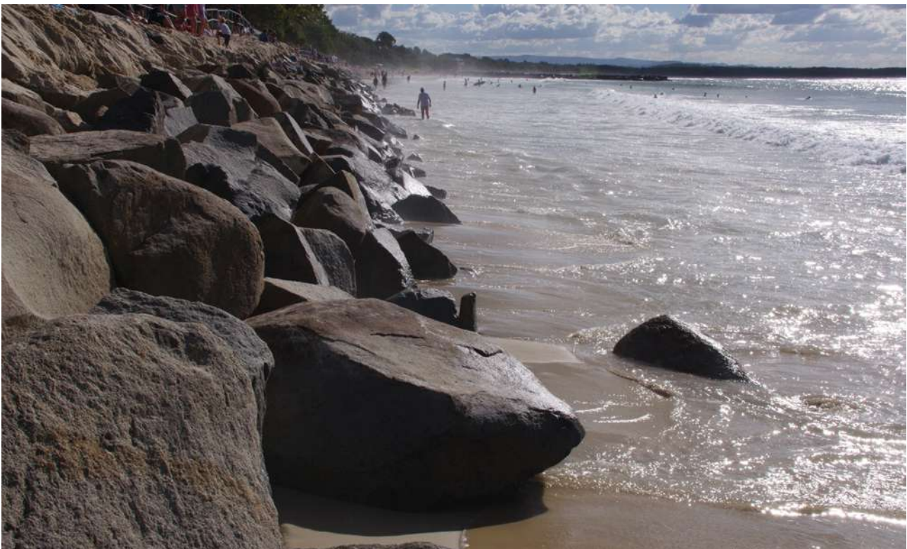
Figure 4.21. Main Beach at Noosa Heads, Queensland, was almost eliminated during storms in the winter of 2019, revealing the underlying rubble defences built in 1969 to protect what is now some of Australia’s most expensive real estate. At this location, natural wave-driven processes can gradually cause the beach to build up again. As in previous such episodes, the approximately 1.3 km long beach was restored by sand pumping and other mechanical measures, estimated to cost AUD500k-750k per annum (Noosa Council, 2018). Photograph by Richard Manasseh.
